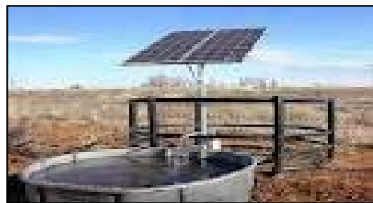
Fig. 1 : A solar pump in open well
